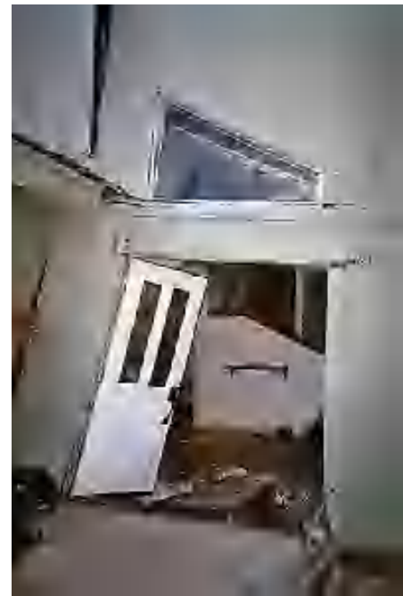
Unbraced cripple walls collapse.
