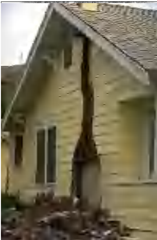
Chimney collapse is a widespread problem.
